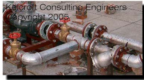
Photo Above: Y-type HVAC strainer incorrectly located on the suction side of pump.
